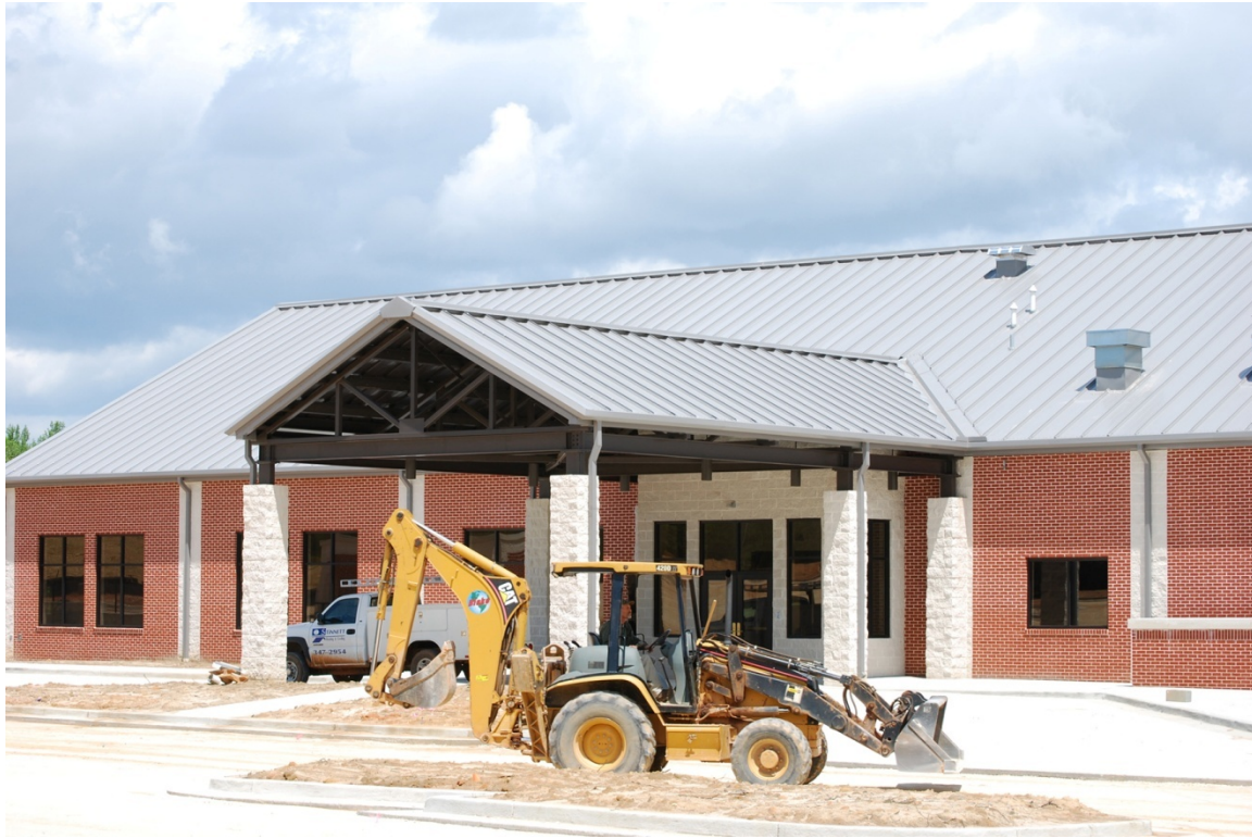
Construction crews work on installing the parking lot at the new fellowship hall of Providence Baptist church on April 20, 2009 at 2900 Lee Road 166.
